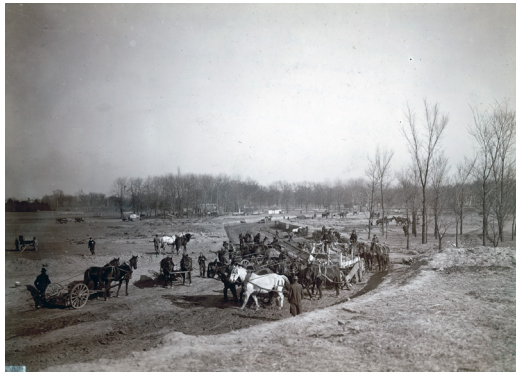
Teams of horses pull excavators and loaders during construction of an excavation channel for the River des Peres in Forest Park in preparation for the 1904 World's Fair. GEORGE STARK. Photo & caption from the MISSOURI HISTORICAL SOCIETY, St. Louis.
