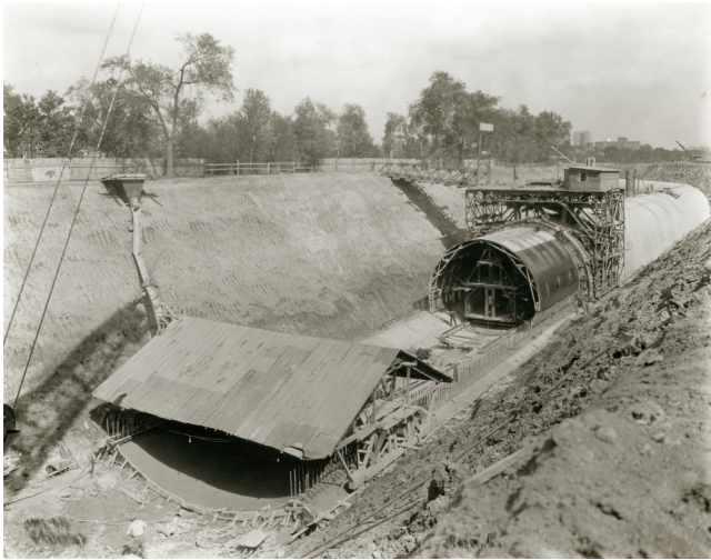
Shelter for pouring thirty-two foot diameter tube in Section E, No. 32 of the River des Peres Sewerage and Drainage Project (near the Jefferson Memorial Building), September 17th, 1929. Photo & caption from the MISSOURI HISTORICAL SOCIETY, St. Louis.
