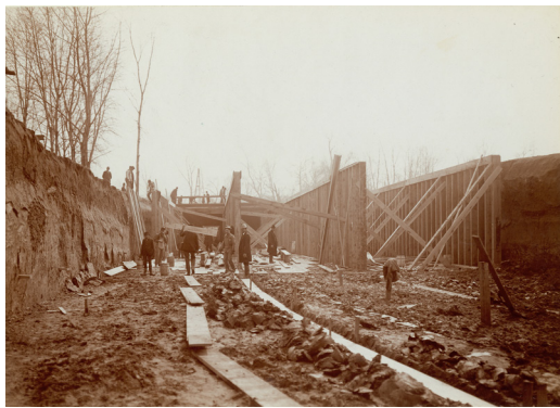
Men at work on a channel way for the River des Peres in Forest Park done for the 1904 World's Fair. GEORGE STARK. Photo & caption from the MISSOURI HISTORICAL SOCIETY, St. Louis.
