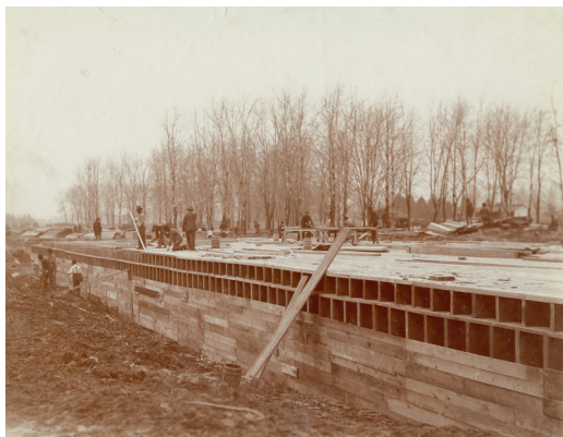
Construction work on a channel way for the River des Peres in Forest Park done for the 1904 World's Fair. GEORGE STARK. Photo & caption from the MISSOURI HISTORICAL SOCIETY, St. Louis.
